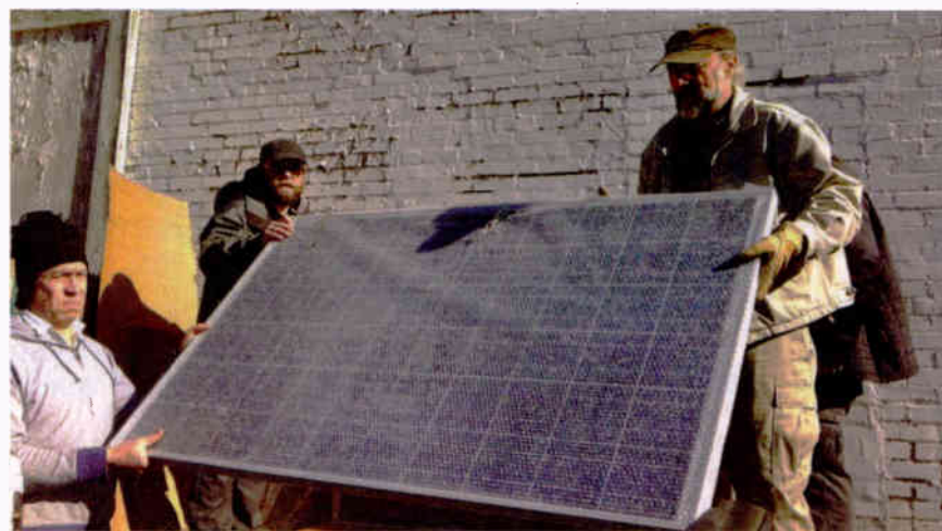
Volunteers prepare to install solar panels on the roof of the KUHS studio building.
