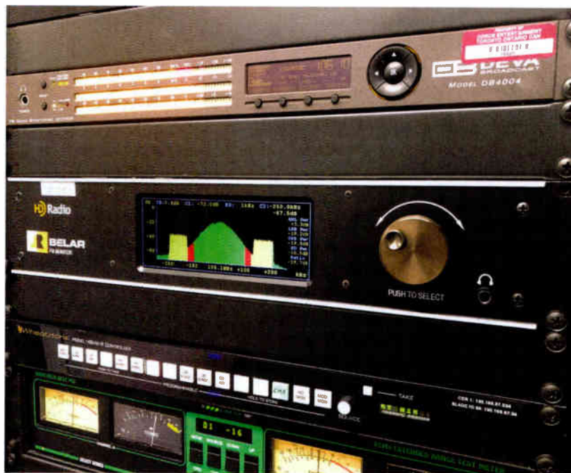
Above The IBOC signal is reflected on monitoring equipment at Corus station CKRY(FM).
