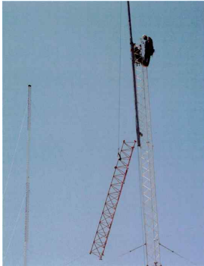
Above Stacking the new towers was easy. Getting to that point was anything but.
