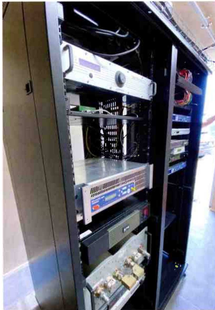
Left An Ecreso transmitter is seen in the middle of the left rack bay.
