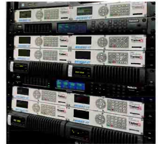
Bridge-IT and Gateway Codecs at MyBridge Radio Network
