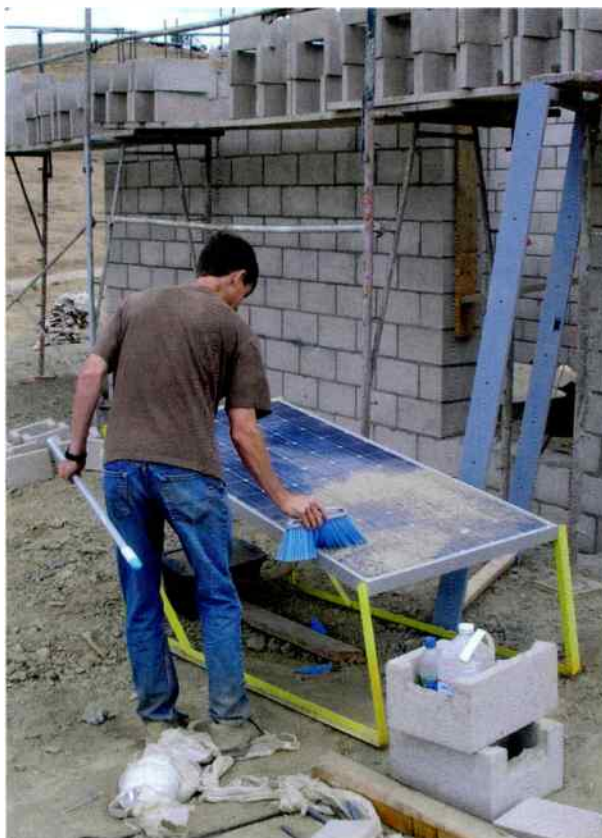
Above Solar power was all we had to run the tower lights during construction at our new Southern California site. Keeping the dust off was a constant chore.
