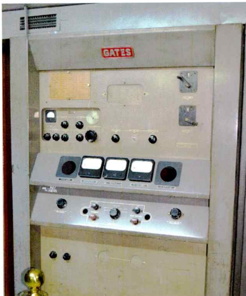
Above A Gates transmitter in the basement of the Saigon Palace.
