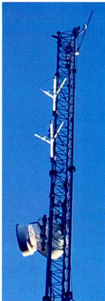
Above This nondirectional Nicom BKG77 antenna serves translator W283BO in Lancaster, Ohio.
