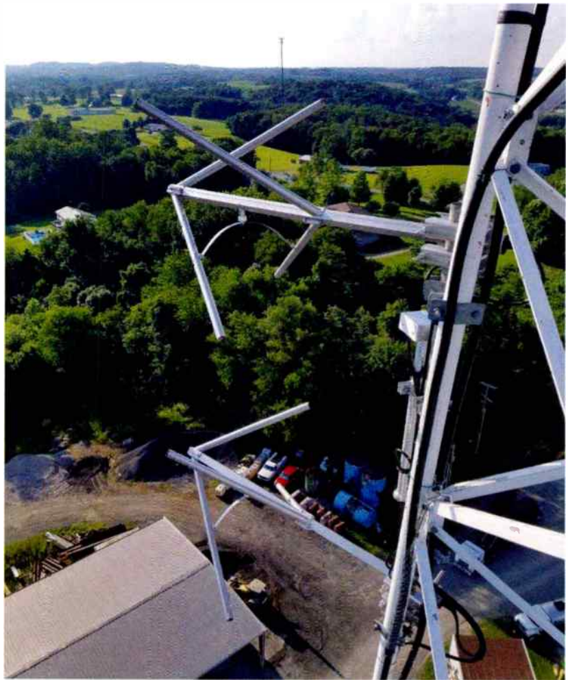
Above A Nicom antenna that translates WLOH(AM) onto 102.9 MHz in Somerset, Ohio. This is configured as a half-wave, "off-the-shelf" directional antenna.
