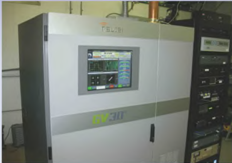
Studio & Transmitter Installation
