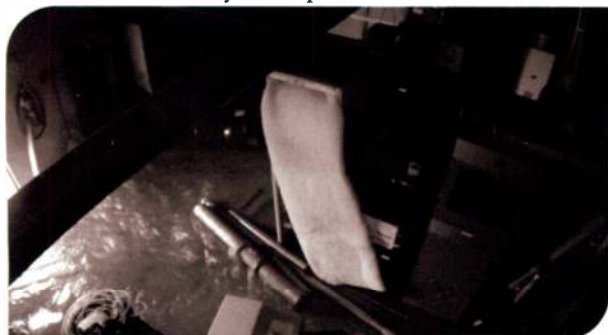
This site's equipment was destroyed by Hurricane Ian. Courtesy of John Clark, Relevant Radio
