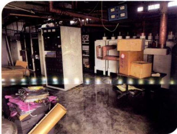
After a fire, smoke and water damage can be more extensive than the fire damage.
