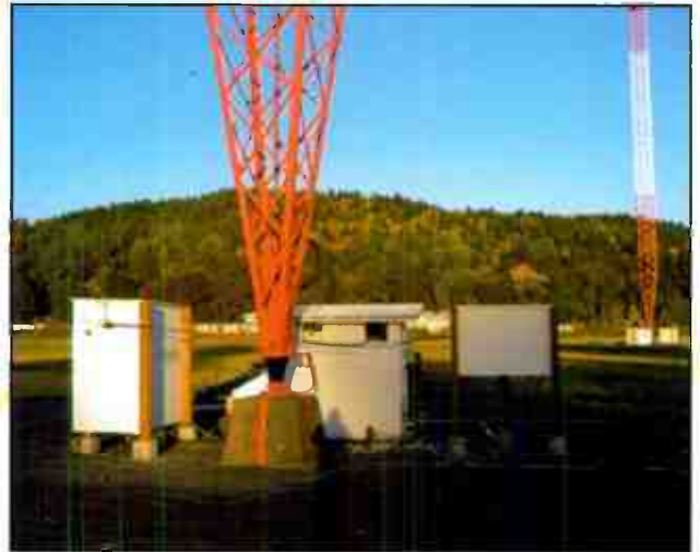
Broadcasters seek rules changes that would affect AM antenna arrays like the one shown here.
