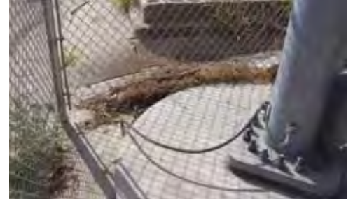
Figure 2. Stranded 250-kcmil bare copper grounding cable connects the base of one studio tower with a buried ring-ground. Note the sturdy mechanical bond at the right.
