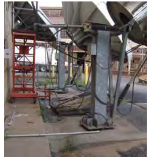
Figure 3. Antennas at the KPTM studio site are grounded with 250-kcmil copper cable protected inside the white conduit. The grounding cables extend from the electrodes and ring-grounds surrounding the towers.
