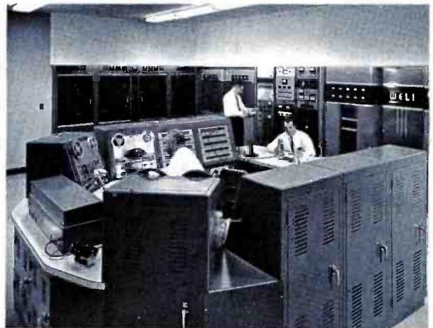
The finest control equipment
