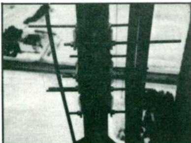
"Splint" over the crack on the present tower leg.
