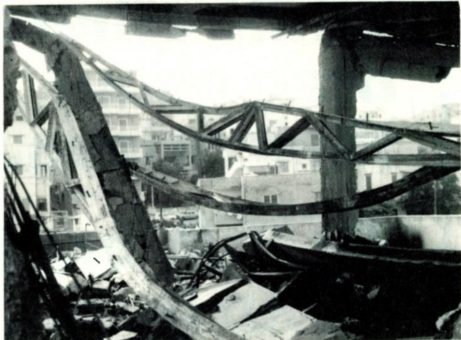
The top floor collapsed at the Far East Broadcasting Association's Beirut radio studio after the building was caught in the crossfire of Lebanon's civil unrest. No one was injured.
