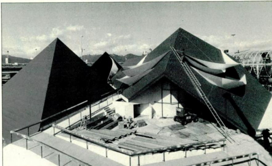
Workmen complete 100 Huntley Street's Pavilion of Promise at Canada's Expo '86. To symbolize peace, the building is designed as a dove with a 60-foot wingspan.
