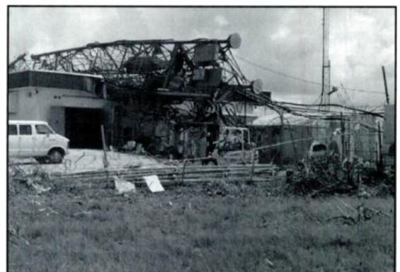
WMCU-FM. WMCU went back on the air September 13 with 18 to 20 percent of its former power. According to station manager Stephen James, full power will not be restored until a new tower is constructed on the old site in about ten to 12 months.
