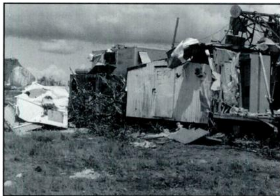
In Homestead, Fla., one of the hardest hit communities, transmitter buildings (photo 1) lie in ruin after Hurricane Andrew toppled WCIX-TV's 1800-foot tower on to the station's building (photo 2). As a result, three Miami-based radio stations were knocked off the air: WXDJ-FM, WRTO-FM, and
