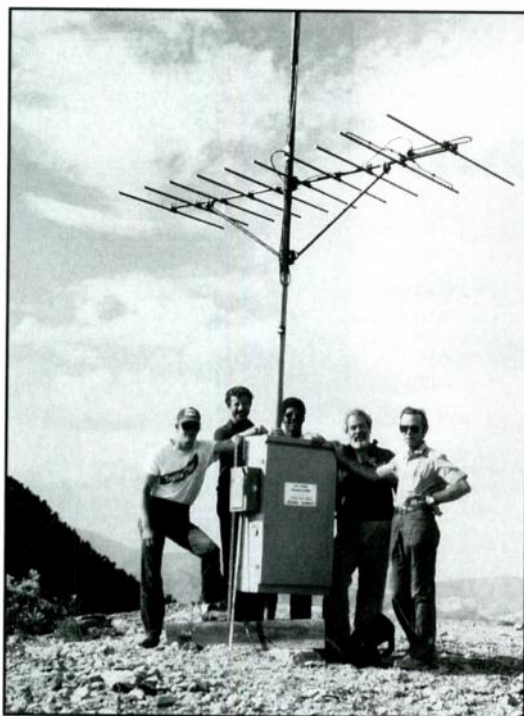
A volunteer pick and shovel crew installed this translator. The cabinet is large enough to accommodate several more translators. Mounted on the pipe is a transmitting antenna.
