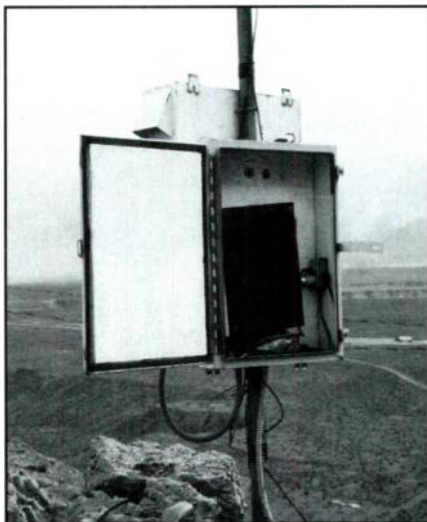
Suitcase translators are housed in the metal cabinet of an FM translator. The translator is located on a mountain to increase coverage and lower both capital investment and operating costs.
