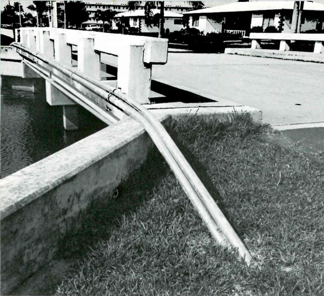
The cable is neatly carried over a culvert. Homeowners may be sensitive to the excavation even when a utility right-of-way exists.
