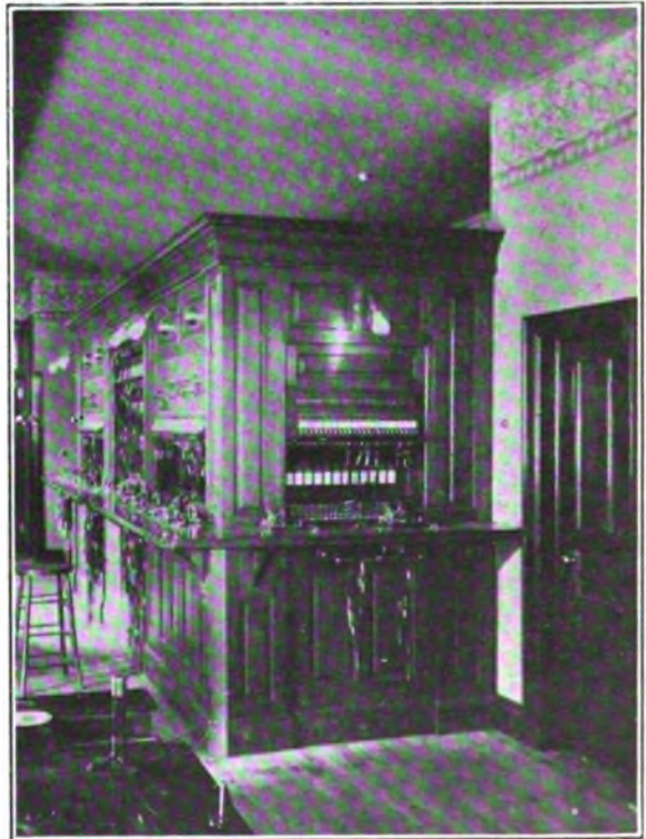
VIEW OF A SECTION OF THE SWITCHBOARD In the Postal Telegraph's New Office, Buffalo, N. Y. and entirely above the switchboard shelf. The feature of interchangeability is of great import-
