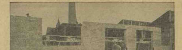
BALLY ENLARGES FACTORY TO PREPARE FOR A BUSY 1940. Photograph shows part of new wing now being rushed to completion.
