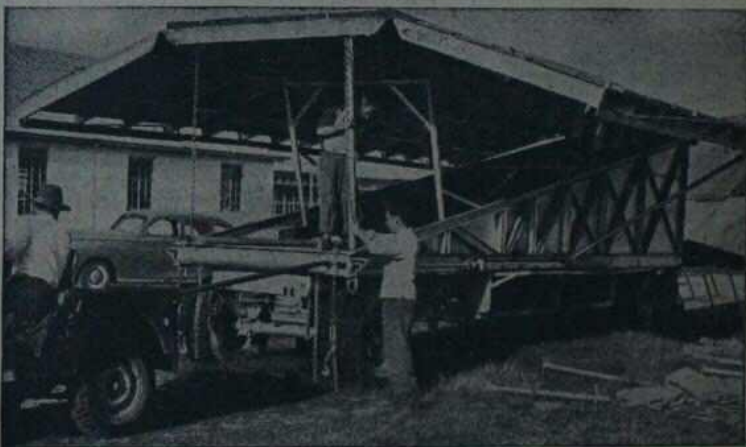
A MOTOR HELPS raise the steel sides while the men place the supports in position. In a very few minutes a complete section is up.
