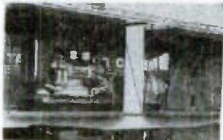
Another view of the world-famous GM Diesel Engine, the controls, and the generator. You can see the chrome on the engine that gives flash and eye appeal. Note the convenience of the junction box.
