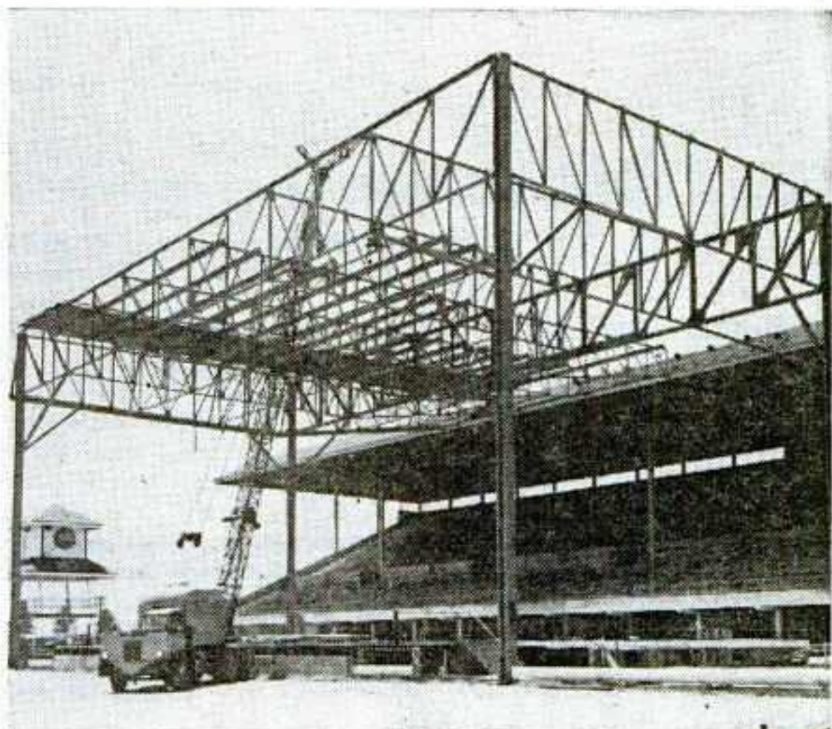
Steel framework for the grandstand stage covering erected this year. Fair spends liberally for top talent; paid Bob Hope $10,000 for one-nighter this year.
