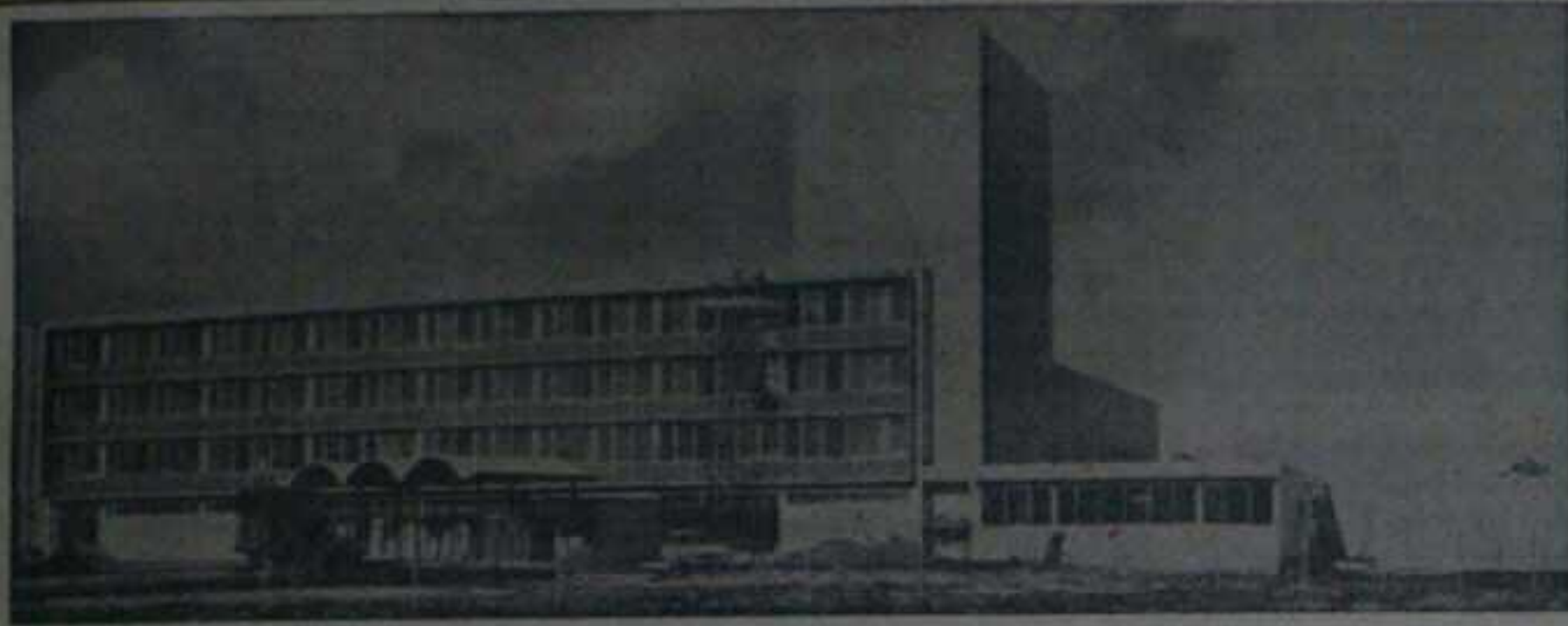
GOTTIEB MEMORIAL HOSPITAL construction is moving into the final phase, as the exterior of the building has been completed. The project should be finished by April 1. The nonsectarian community hospital, in a West Chicago suburb, was initiated four years ago by David Gottlieb, prominent game manufacturer, whose family foundation contributed more than $750,000 for the 120-bed institution. First scheduled event in the new building was Wednesday (20) when 200 businessmen and staff physicians heard progress reports.
