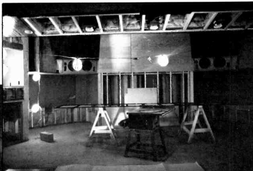
Pierce Arrow Recorders in Evanston, Ill., under construction. When completed it will house two studios, a mixing room and mastering room. Says manager Frank Seater, "They've provided a bang-up foreman and great plans. They've even helped us with our own financial presentations."
