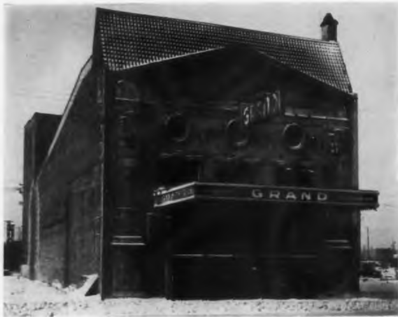
When jazz came up from New Orleans to Chicago, one of the places in which it found a home was the Grand Theater at 3110 S. State St. Here, the Grand is seen as it goes under the wrecker's hammer. The historic landmark is being demolished by the Chicago Land Clearance Commission to make room for a redevelopment project near the Illinois Institute of Technology.
