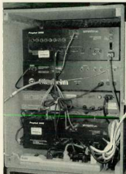
FIG. 2: A properly wired rack.
