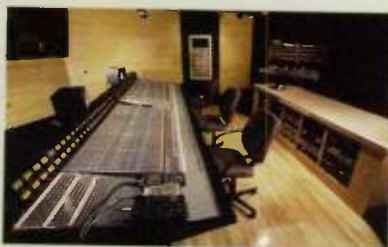
S.S.L. 4080 G plus with Ultimatum Control Room 2
