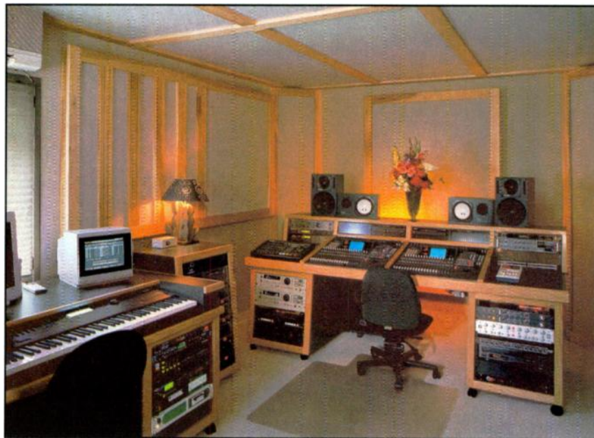
Christopher Cross's personal studio. Notice how sound absorbers are strategically placed on the walls and ceiling as well as in the corners.
