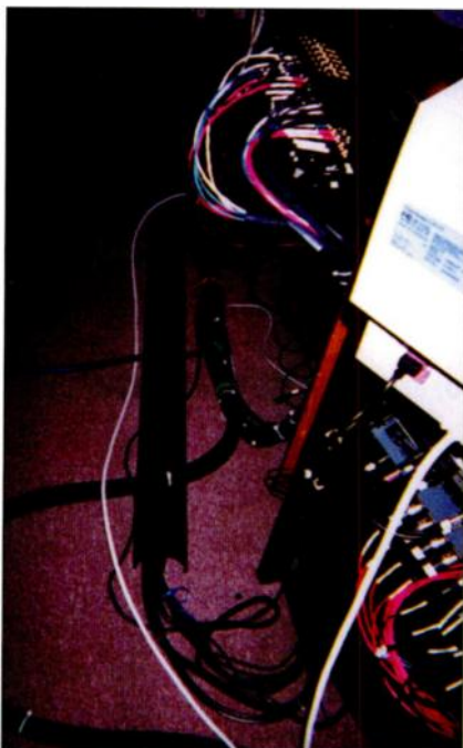
FIG. 6: This cable bridge protects cables from foot traffic at Toys in the Attic. Note that separate cable bundles from different stations are joined together, and analog audio passes at a right angle over the digital-audio run.
