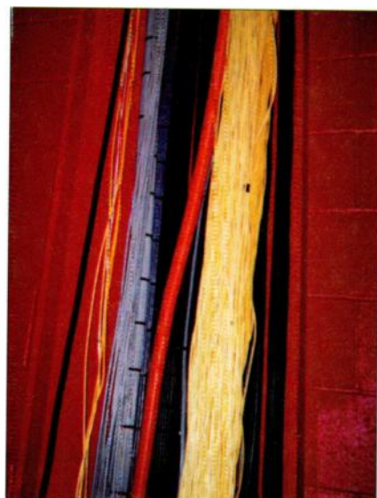
FIG. 5: In the Ex'pression Center for New Media's central machine room, managed cables and bundles cascade down a chute from a raceway in the ceiling to a trough beneath the floor.
