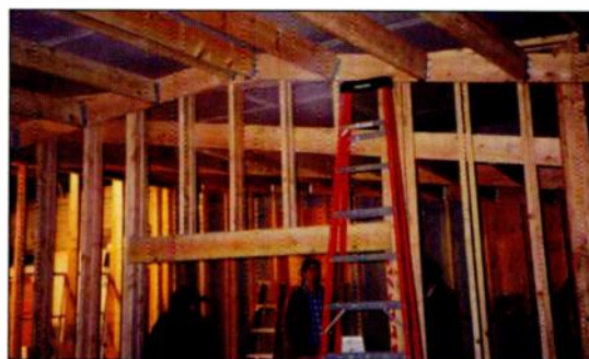
FIG. 6: If you own the building that houses your studio, you will have greater freedom to substantially alter its physical structure, which might include changing a room's shape to enhance its acoustical properties.
