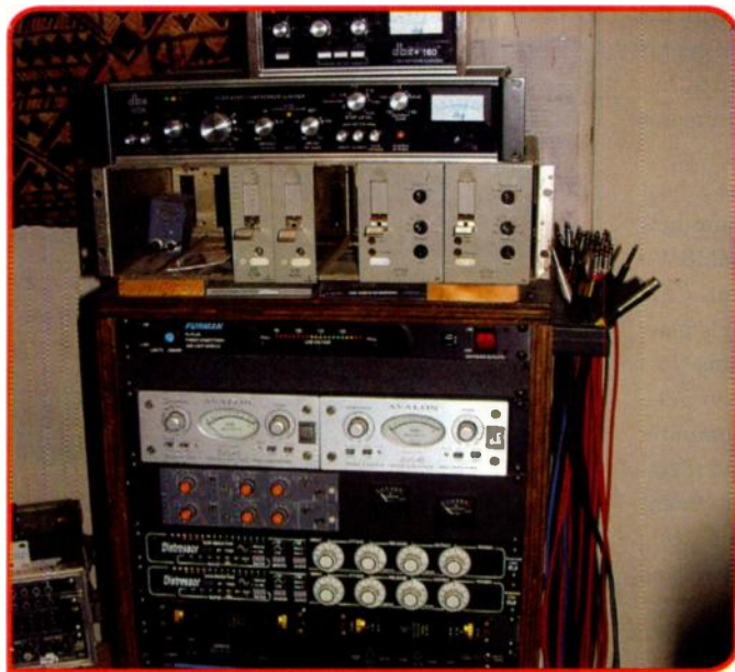
FIG. 4: The control room rack at Shacklyn features outboard gear from Avalon, dbx, Empirical Labs, Furman, Lexicon, Neve, Telefunken, and Yamaha, among others.
