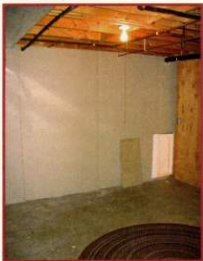
FIG. 1: An unfinished basement is an ideal place to build your own echo chamber.
