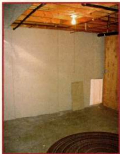
FIG. 1: An unfinished basement is an ideal place to build your own echo chamber.
