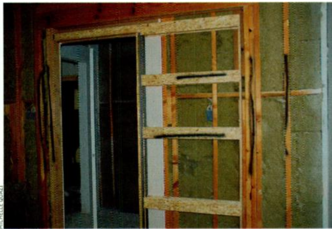
FIG. 4: This photograph was taken during construction of Vole Studios. The walls are made of recycled wood, with mineral board used for insulation. No virgin wood or fiberglass was used.
