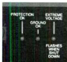
You always know your power and protection status before your equipment is switched on
