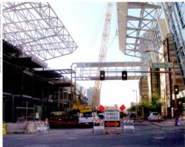
THE "GOLDEN SPIKE" of the Phoenix Convention Center expansion project – a bridge that connects the new "West Building" with the new "North Building" – is lifted into place January 22nd.
