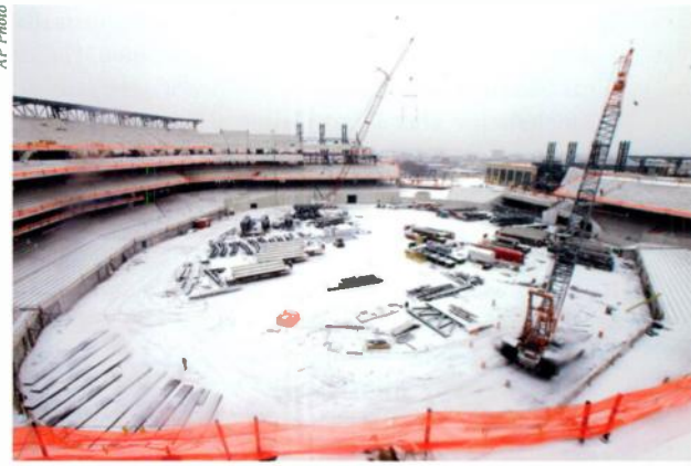
CONSTRUCTION WAITS FOR A THAW AT CITI FIELD, the site of the new baseball stadium for the New York Mets in the Queens borough of New York City. The $800 million project is on course for a January 2009 debut.
