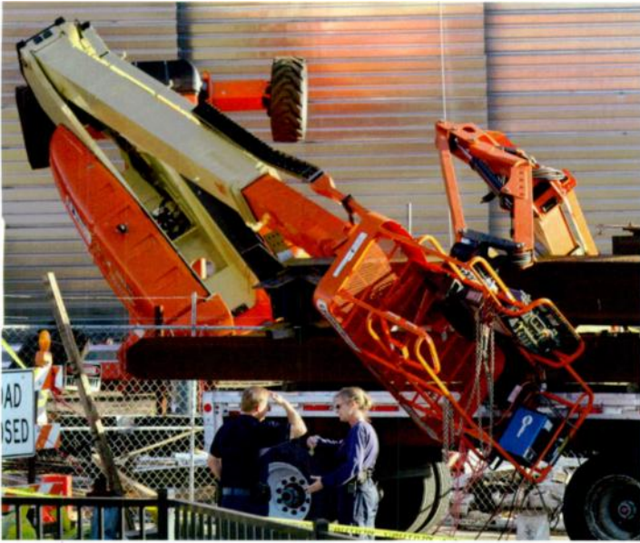
AUTHORITIES INSPECT A PORTABLE BOOM LIFT that fell over at the construction site of the Kauffman Center for the Performing Arts in Kansas City, Mo., Nov. 10. Local and federal investigators are trying to determine what caused the accident that killed one worker and left another in serious but stable condition.
