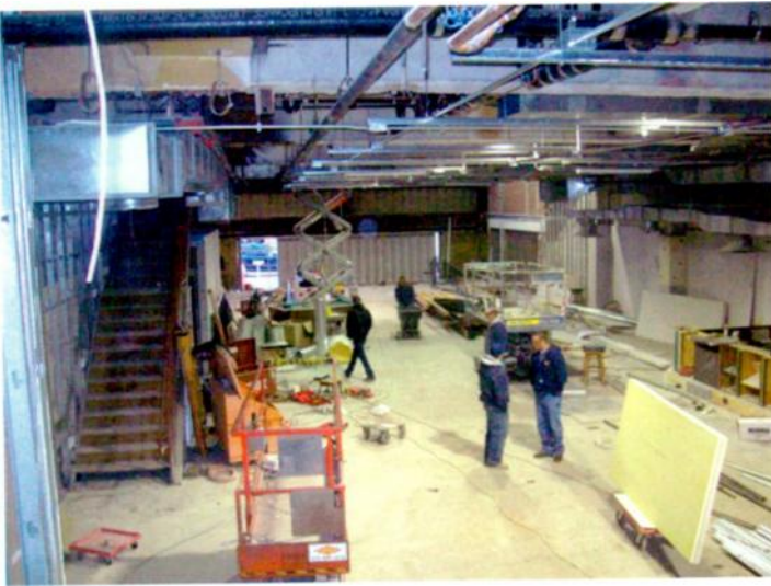
CONSTRUCTION IS IN FULL SWING at the newest Knitting Factory location in Reno, Nev., Nov. 19. The remodeled venue is scheduled to open Jan. 1.
