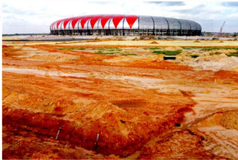
CONSTRUCTION CONTINUES D-c. 14 on one of the stadiums that will host the 2010 African Cup of Nations soccer tournament in Angola, which will host the event in January.
