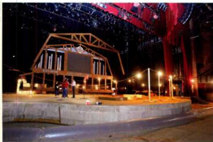
HEAVY FLOOD DAMAGE TO THE GRAND OLE OPRY HOUSE in Nashville led to workers tearing out sections of the building down to its concrete foundation May 13 so repairs can be made.
