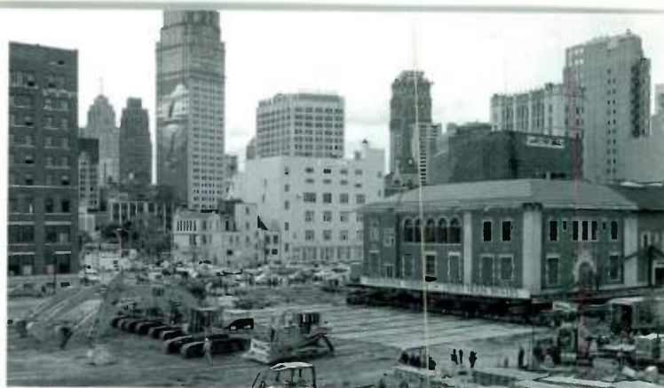
TWO BULLDOZERS with cables anchored to four excavators are used to start the Gem Theatre on its way to its new location.
