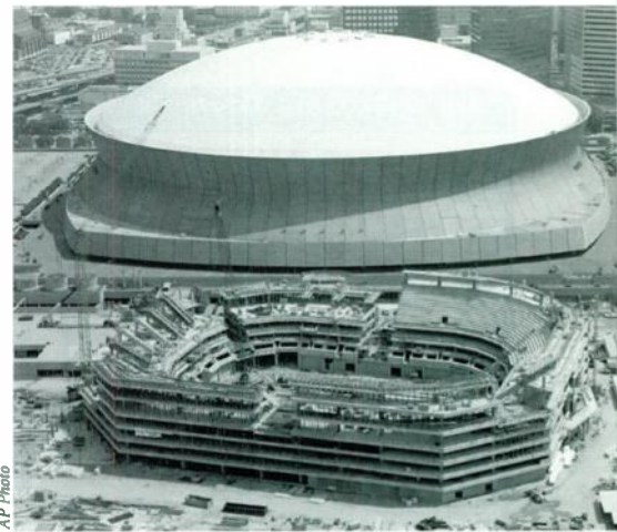
CONSTRUCTION CONTINUES on the new sports arena being erected next to the Louisiana Superdome in New Orleans. The Superdome Commission voted May 13th to recommend that the New Orleans Brass hockey team be awarded the lease to the venue.
