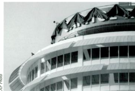
WORKERS PLACE black bunting atop the Capitol Records tower in Hollywood in tribute to the Chairman of the Board.
