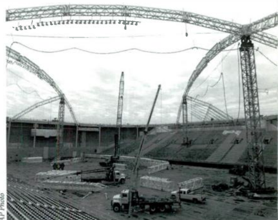
STILL WITHOUT A ROOF , the UNI Dome at the University of Northern Iowa continues to undergo construction to replace the venue's air-supported dome. As shown here June 6th, most of the stainless steel supports are in place, which will hold the stadium's new fabric roof.
