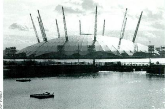
THE ROOF is up on the Millennium Dome . The British government hopes the massive structure on the River Thames will raise the U.K.'s profile as a happening place.
