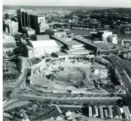
EXCAVATION IS COMPLETED at the site of the new Saint Paul Arena. The old Saint Paul Civic Center was torn down to make room for the new multipurpose venue, which will be home to the NHL's Minnesota Wild. The $130 million facility is scheduled to open in October 2000.
