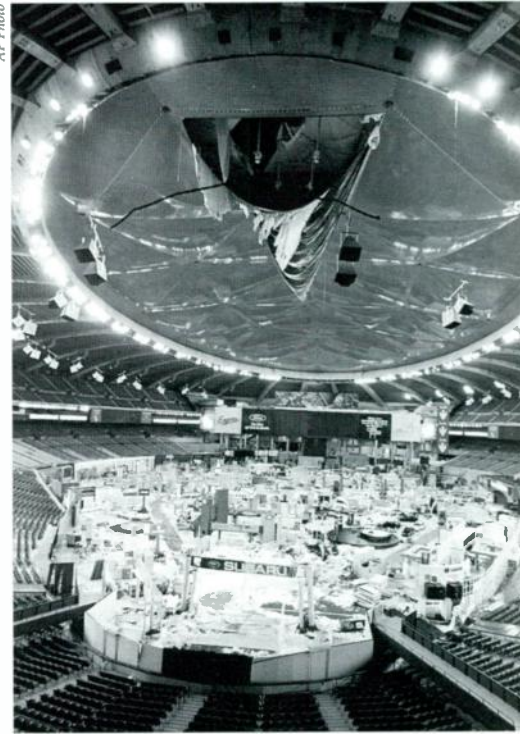
WATER POURS THROUGH a hole in the new roof covering Montreal's Olympic Stadium.
